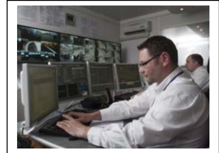
Figure B-5: Heathrow Control Room.
